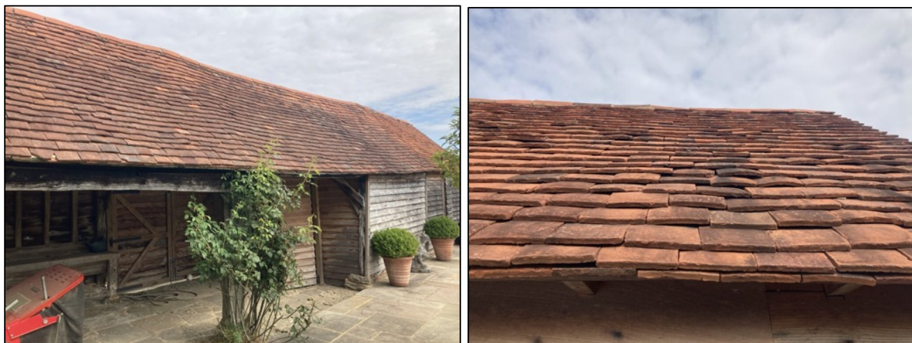
Photograph 6a & 6b. The southern pitch (left) of the covered walkway at Town House Farm, with examples of the gaps under the roof tiles on this section (right).
