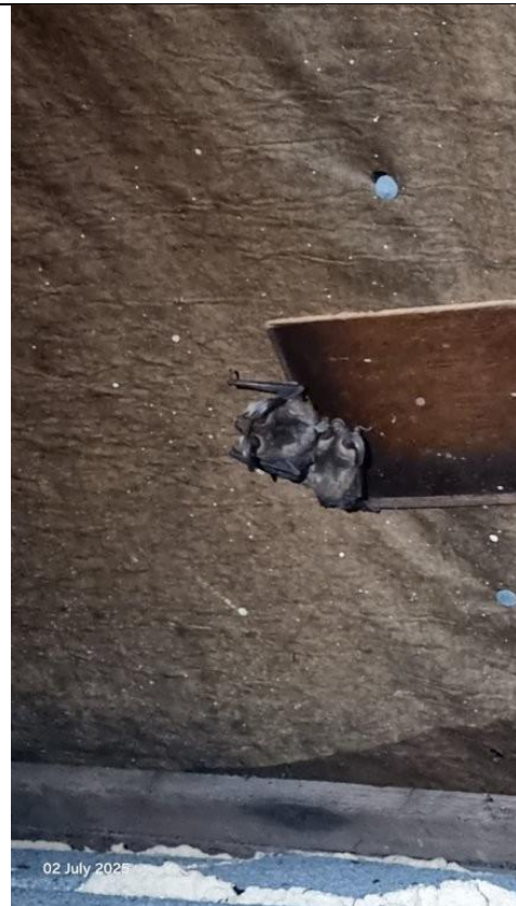
Plate 12. Bats in crawl space
