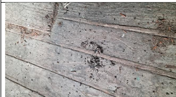
Plate 7. Bat dropping in Outbuilding 1
