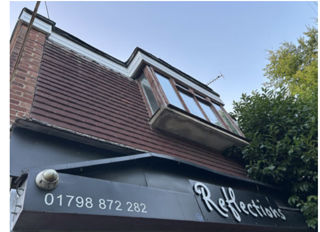
Figure 1a: Hanging tiles and soffits on southeastern elevation of B1.
