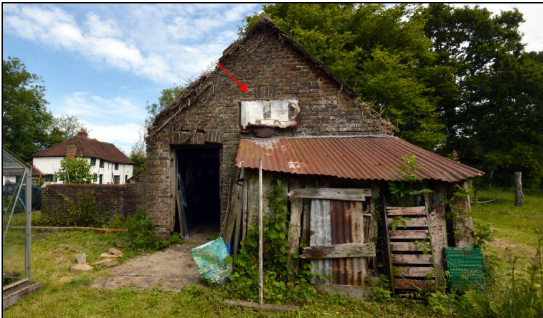
Plate 12: The south end of the group with the surviving voussoirs indicating the location of the original gable window (arrow)
