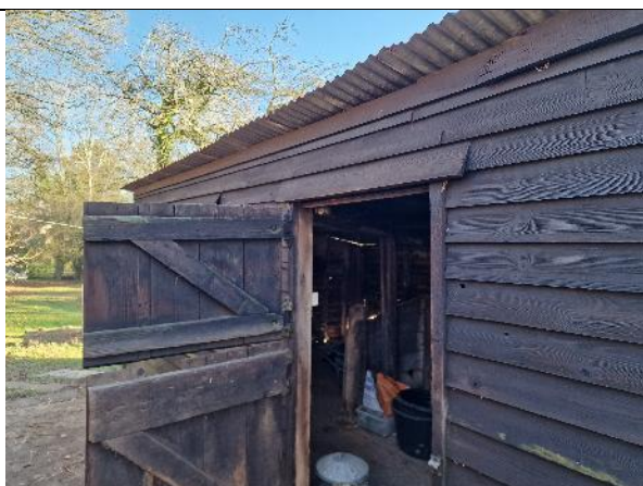
Building 2. Front view, access to internal space via gaps in doors and roofing.
