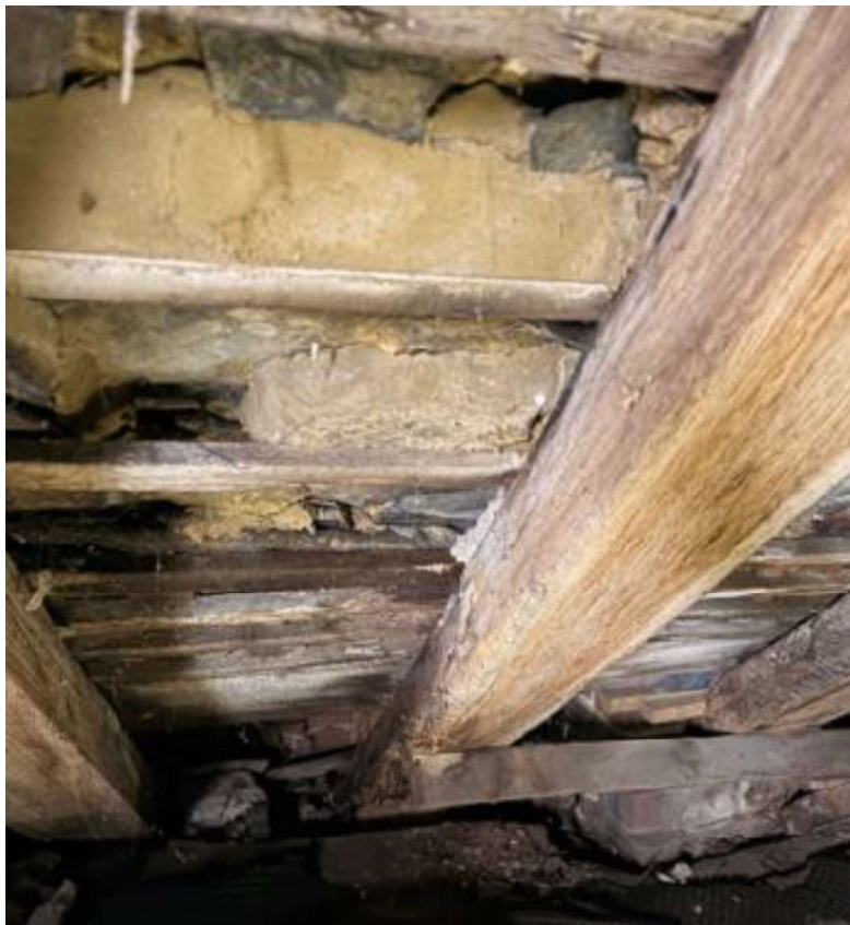
ROTTEN ENDS TO 4 & 5 – ADD STEEL PLATES
