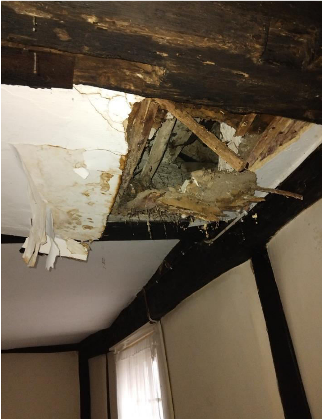
Figure 9: The section of ceiling within the eastern part of the building at first floor level that has suffered severe damage due to water ingress and structural issues from the loft space above.
