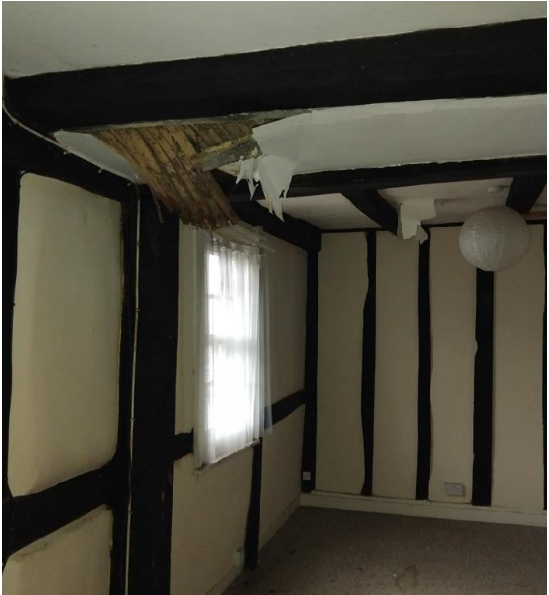
Figure 10: Different view of the section of ceiling within the eastern part of the building at first floor level that has suffered severe damage due to water ingress and structural issues from the loft space above.
