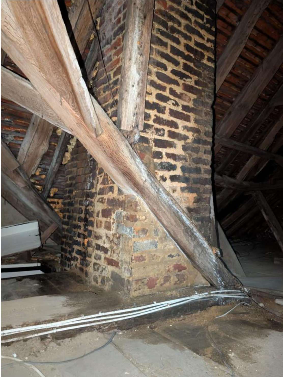
Figure 7: Visible water ingress to the chimney stack.
