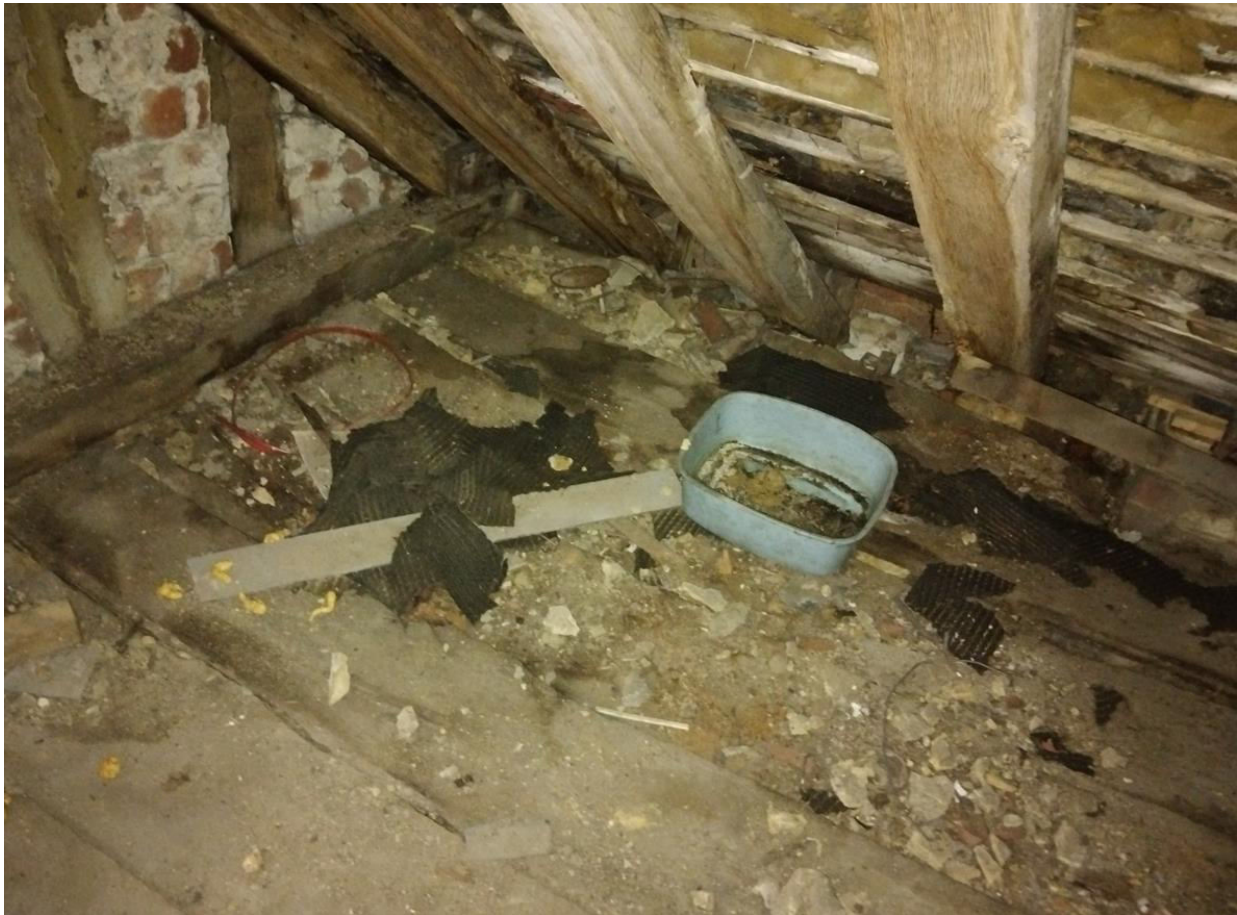
Figure 5: Visible water ingress within the south-east corner of the loft space.
