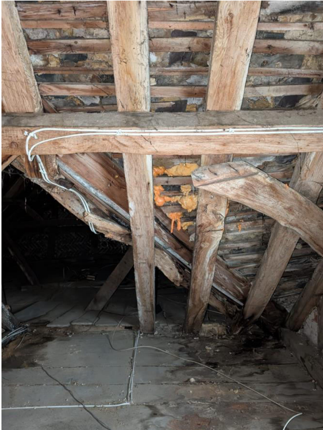
Figure 6: The damaged timber elbow and damaged valley board.
