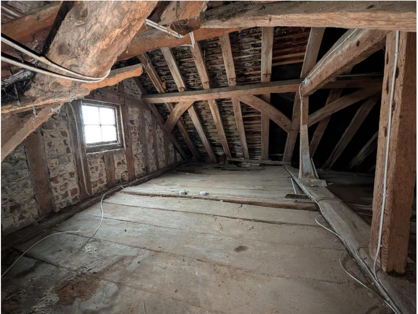
Figure 5: The existing loft space showing the south facing rafters that require steel plates to be fitted. There is evidence of water ingress in this location.
