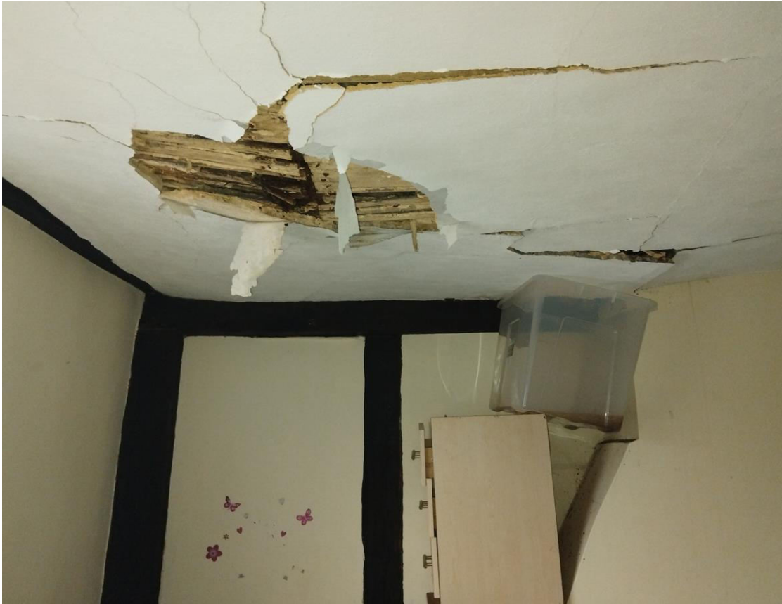
Figure 11: The section of ceiling within the south-eastern part of the building at first floor level that has suffered severe damage due to water ingress from within the loft space above.
