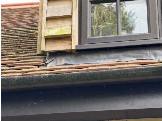
Example of potential ingress point.
