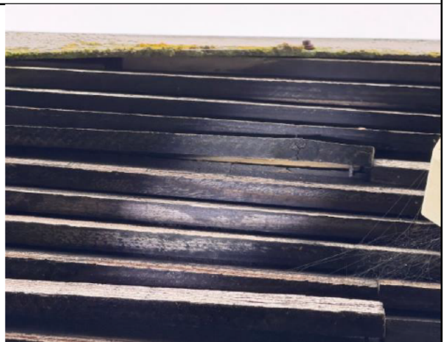
Photograph 18: Gaps underneath the timber cladding on the southern elevation.
