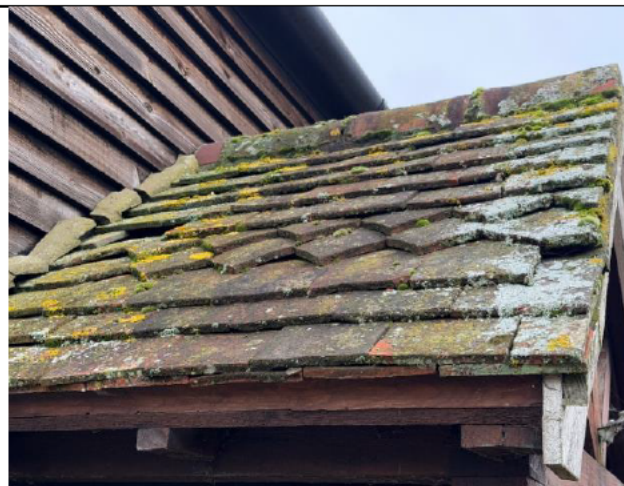
Photograph 19: Missing tiles on the porch canopy.
