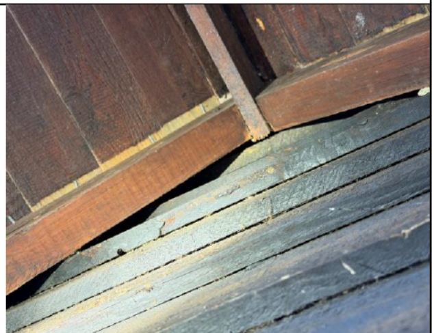
Photograph 20: A gap between the porch canopy and timber boarding.
