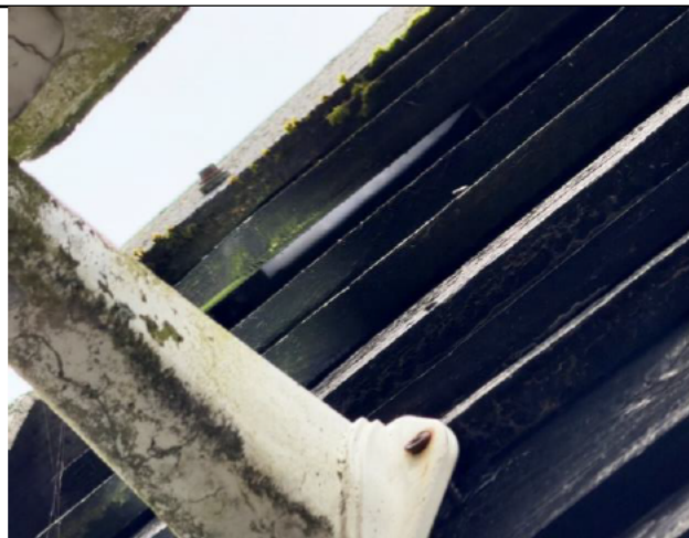
Photograph 17: Gaps underneath the timber cladding on the southern elevation.
