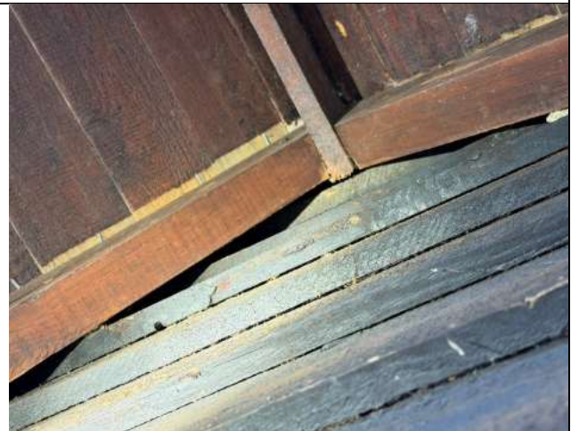
Photograph 20: A gap between the porch canopy and timber boarding.
