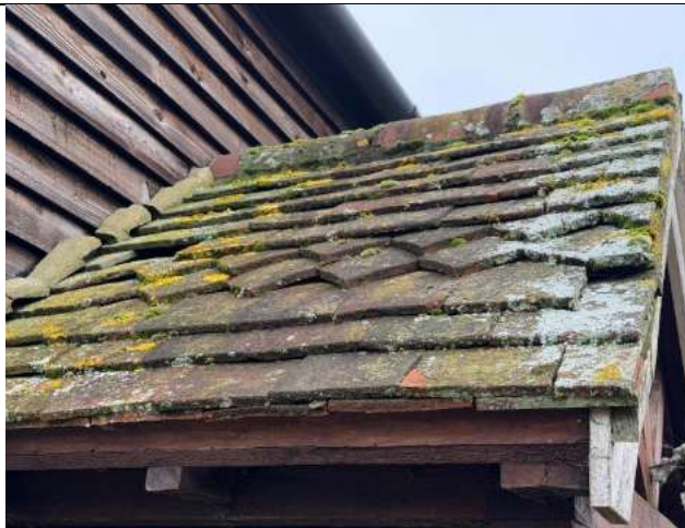
Photograph 19: Missing tiles on the porch canopy.
