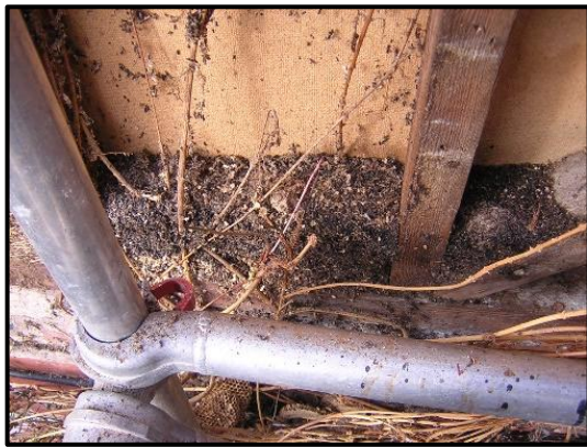
Pipistrelle droppings in exposed wall cavity
