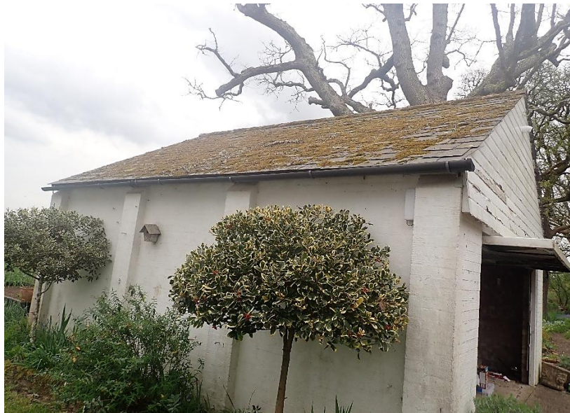
Fig. 4 – Garage, viewed from the north – moss covered slates on roof
