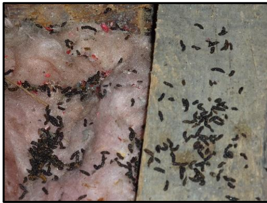
Long-eared bat droppings in roof void
