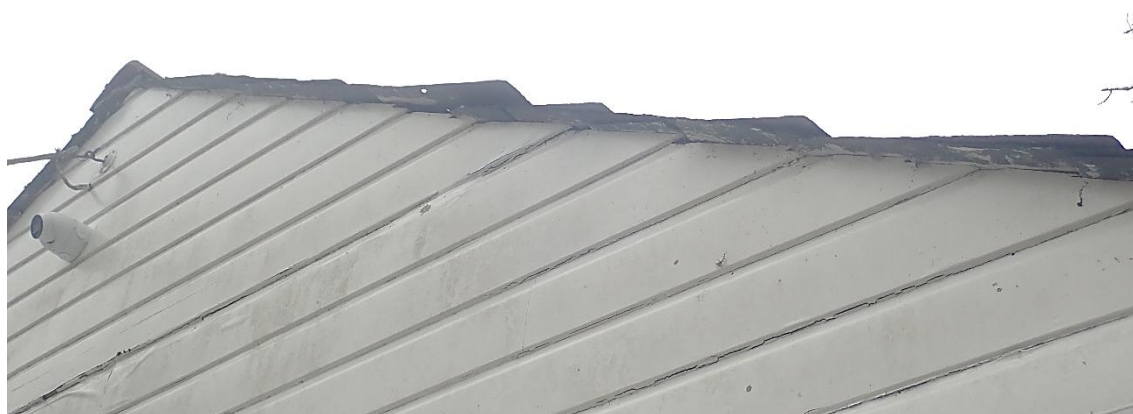
Fig. 8 – Slipped slates on roof verge
