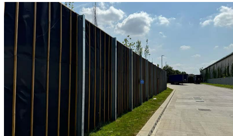
Acoustic Fencing - 1.8m height
