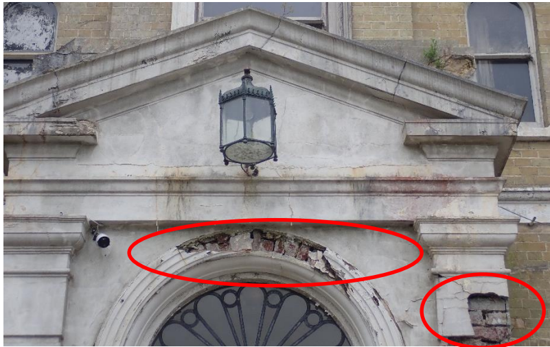
Fig. 3 – Examples of damage to plasterwork (Main entrance, north-east of house)
