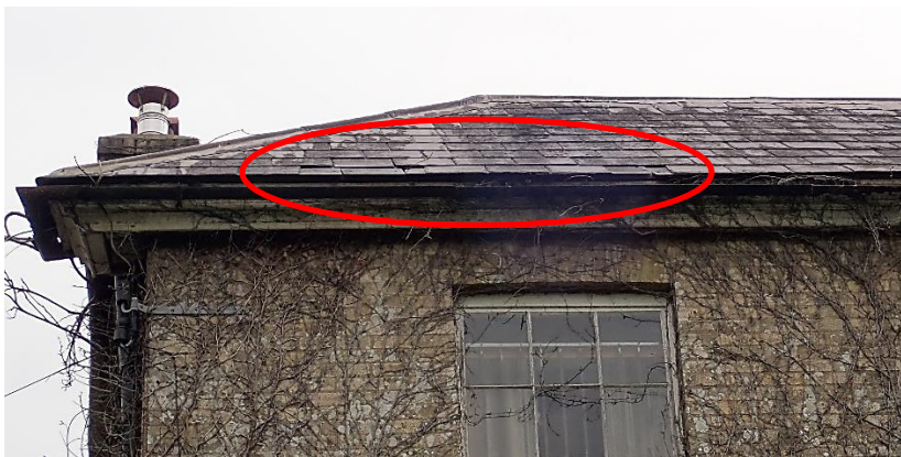
Fig. 2 - Example of slightly uneven slates on roof (north-east of house)
