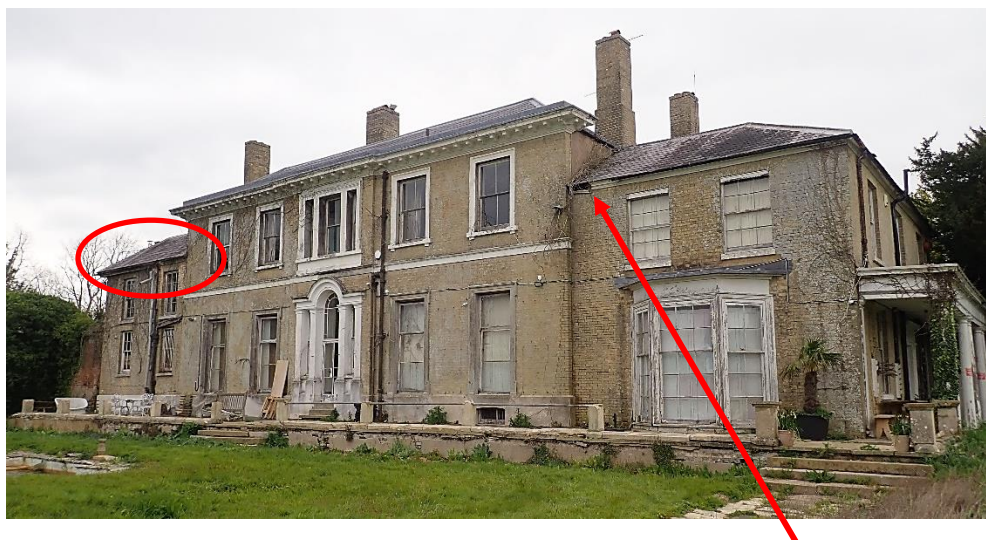
Fig. 5 – Rear (south) side of house – SW roof (not searched) circled. Area of damage at eaves level
