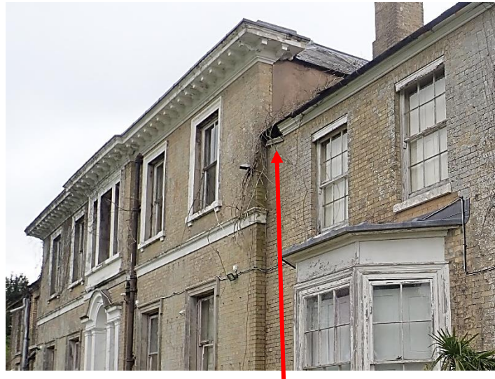
Fig. 6 – Rear (south) side of house – area of damage at eaves level, closer view
