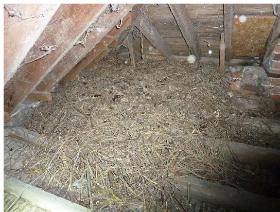
Fig. 10 – jackdaw nest in roof void
