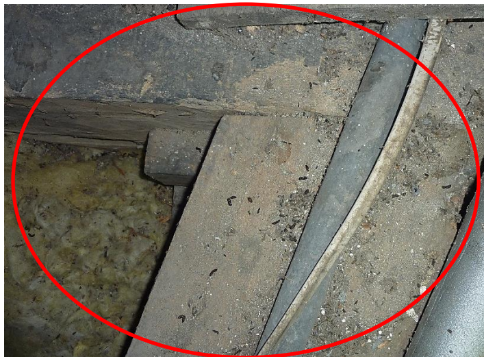
Fig. 9 - Small number of bat droppings in Roof Void 3
