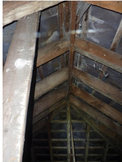
Fig. 8 - Unlined Section of roof
