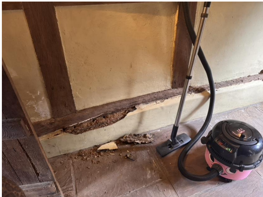
Photo (ix) – small section of mortar removed revealing decayed ground beam
