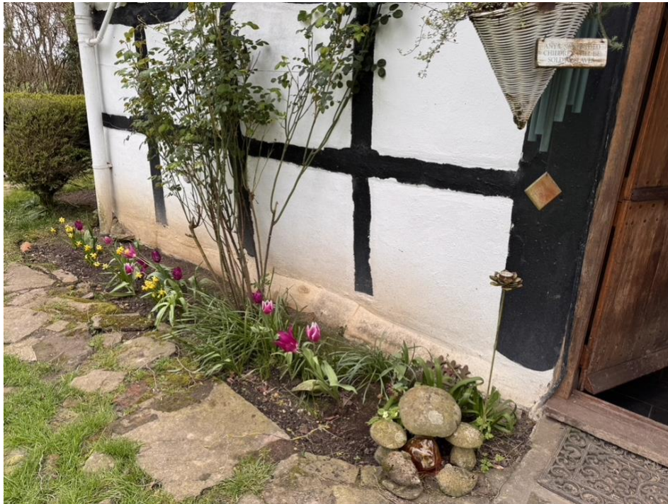
Photo (xi) – ground beam encased in cement render to be replaced
