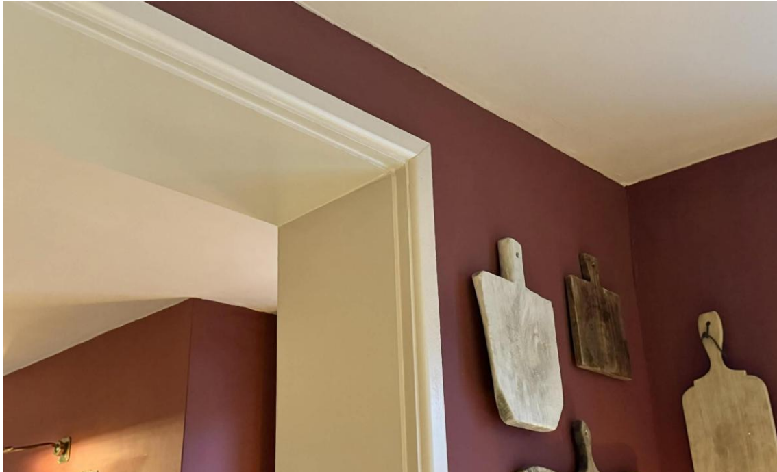
Fig 3: Large nibs and a ceiling beam have been left at each side, showing the outline of the original wall. Whilst the loss of historic fabric cannot be condoned, anything that replaces it can only ever be a replica and the existing side nibs and ceiling beam do at least broadly continue to allow for the appreciation of the former divide to be still clearly understood.
