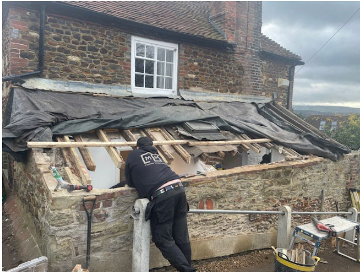
Plate 25: Timber rafters of different sizes prior to works with rotten roof timbers visible.
