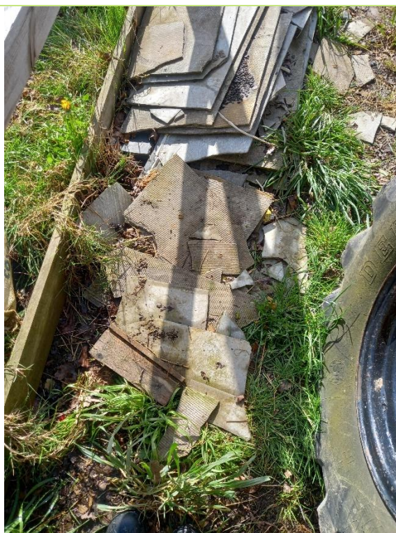
Photo 16- Possible ACM in yard area.
