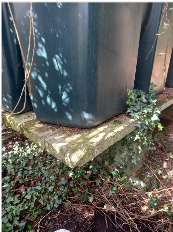
Photo 2: Oil tank on Plinth
