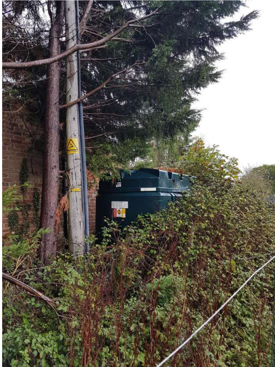
Photo 20: Double-skinned, banded, oil tank behind main residence. Note the diagonal cracks in brick in background.
