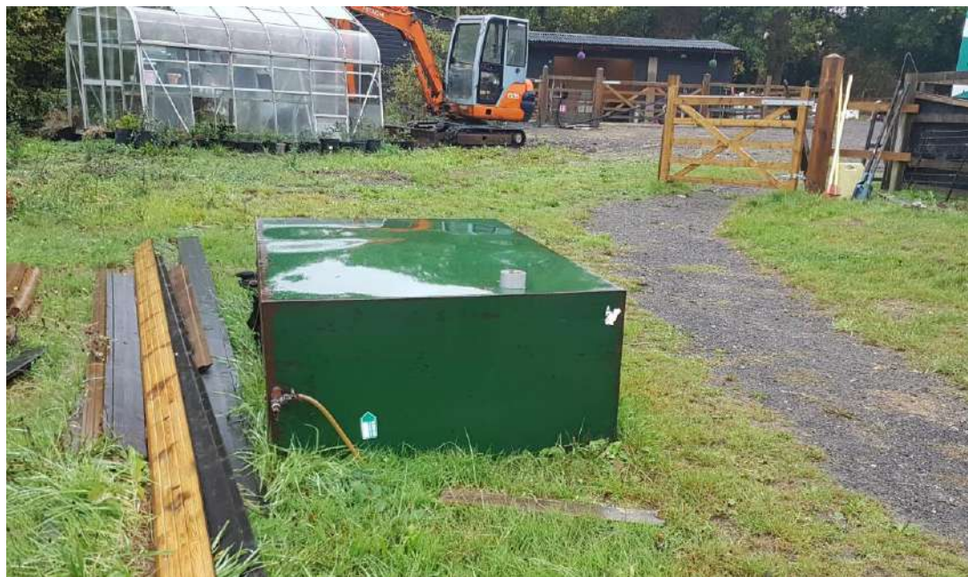
Photo 9: Single skinned, unbunded and disused oil tank near static home.
