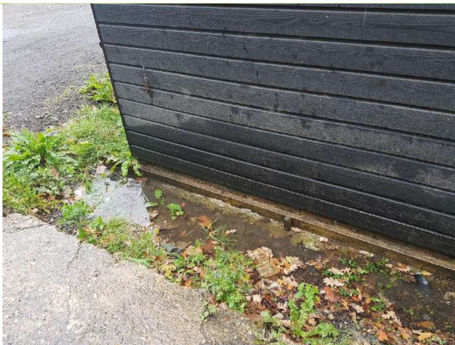
Photo 4: Water pooling in drainage ditch around stables
