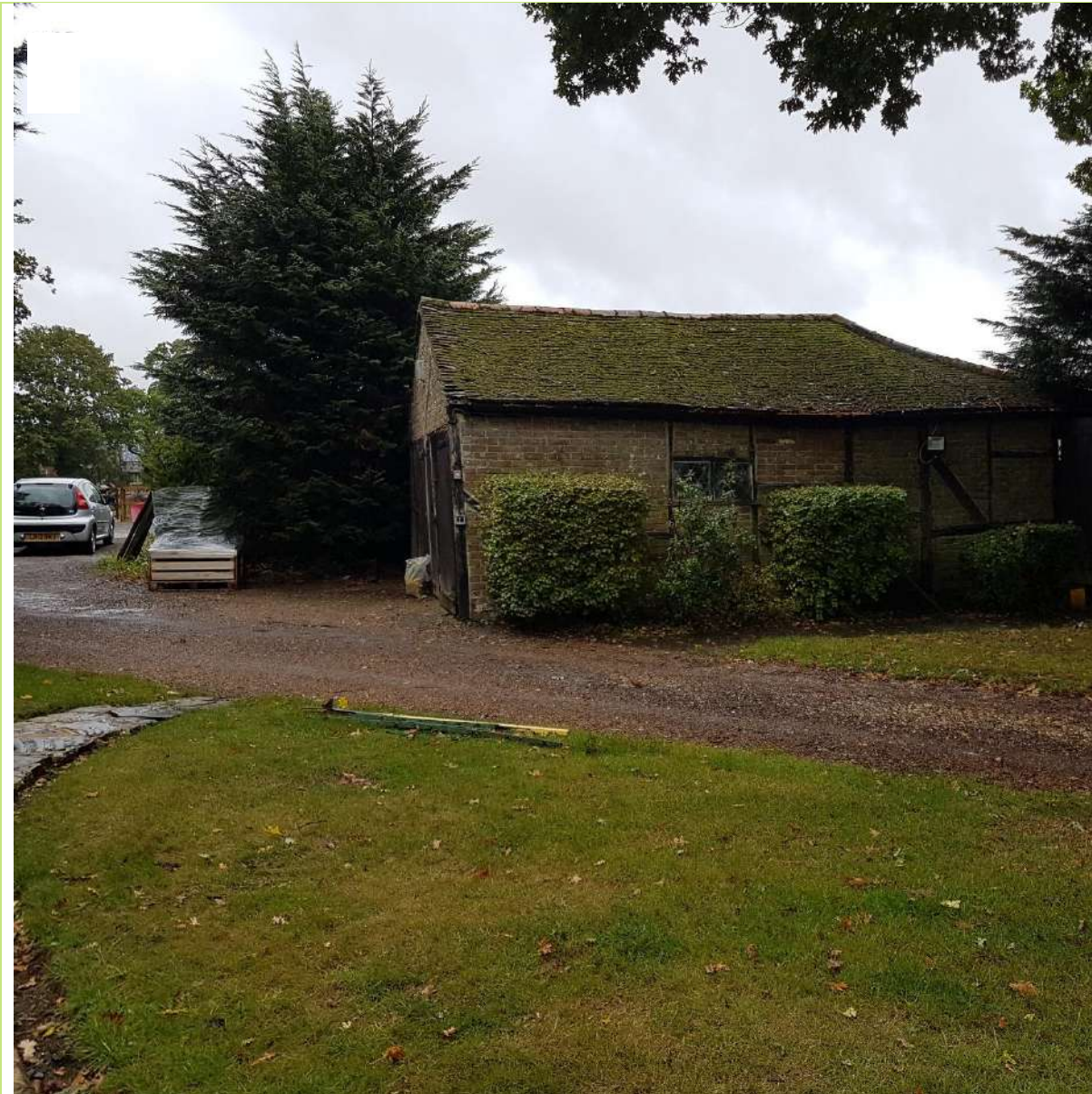
Photo 23- Storage building attached to stables, note appearance of sunken roof and out of alignment walls.
