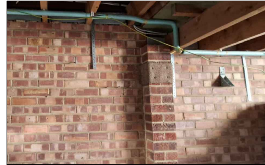
7 - Flat roof joists Level difference
