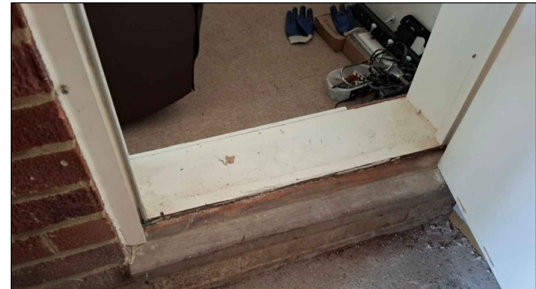
8 - Floor level difference between garage & house
