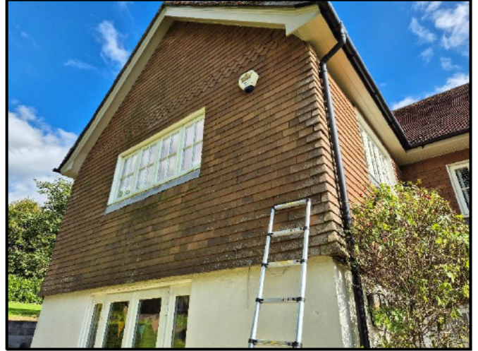
Photo 6: Gable of hanging tiles affected..
