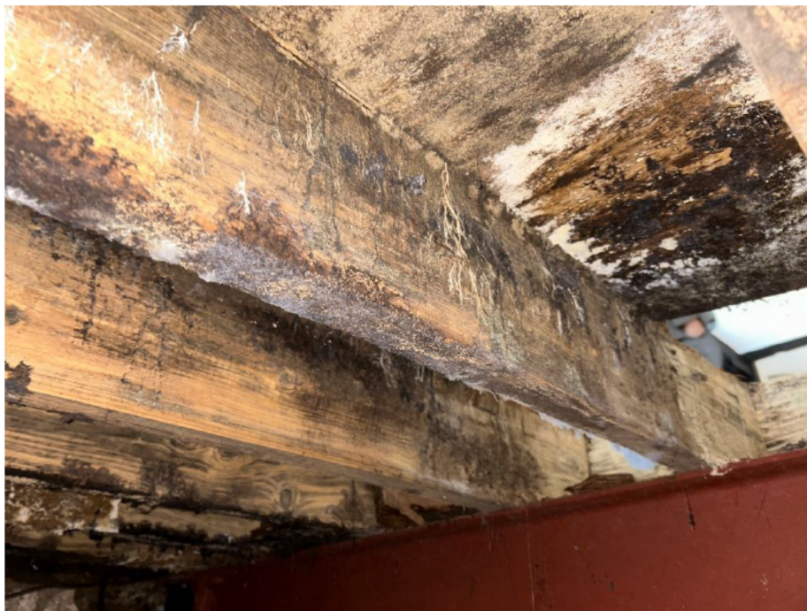
Photo 12: Existing floor joists affected by dry rot
