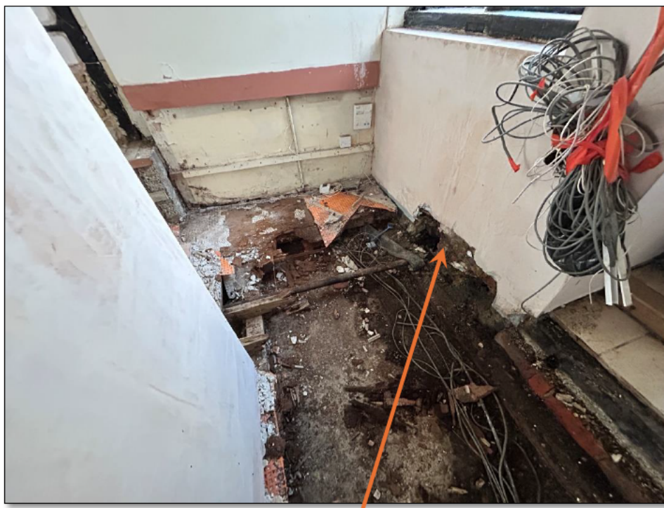
Photo 5: Damage timber flooring removed & source of leaking pipe exposed.
