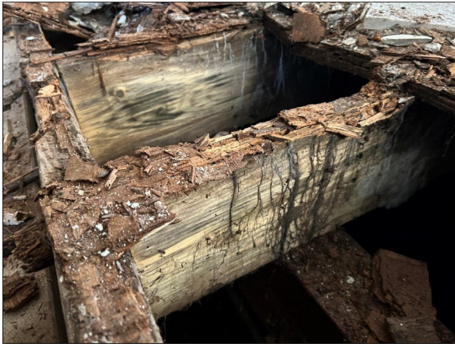
Photo 7: Decayed timber floor joists
