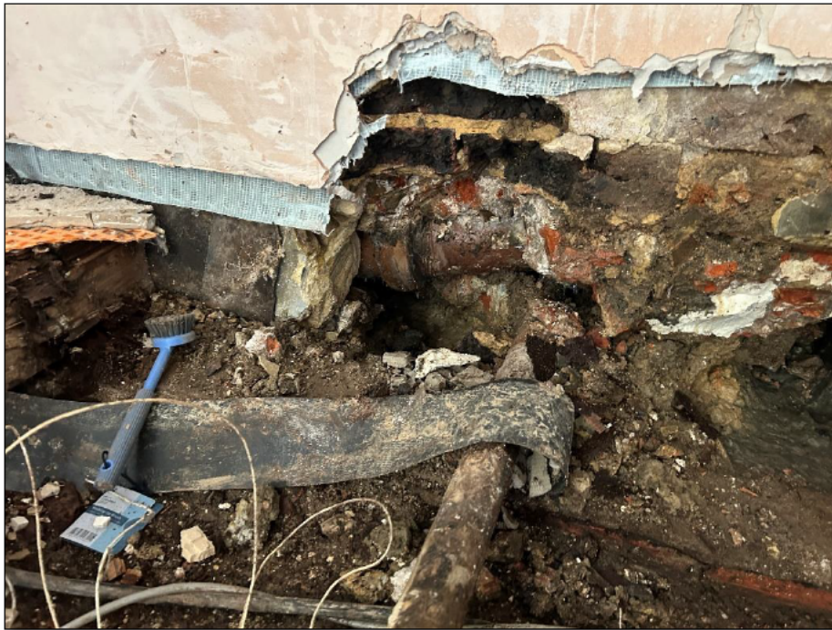
Photo 4: Wall exposed internally to reveal defective pipe in wall.
