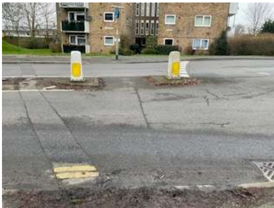
Figure 2: Ponding and detritus at crossing point.
