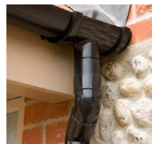
Black rainwater goods
