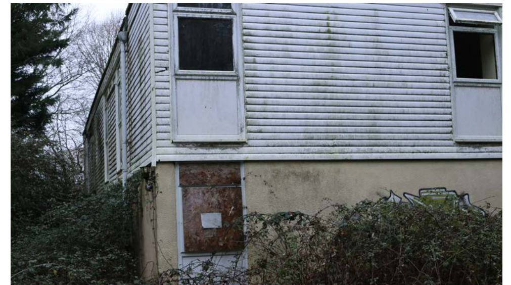
Site Photograph E. Poor state of repair of built form on Site.
