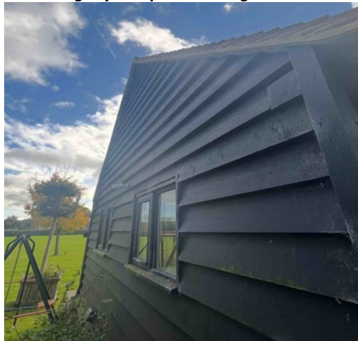
Plate 3: Slightly Warped Cladding Boards
