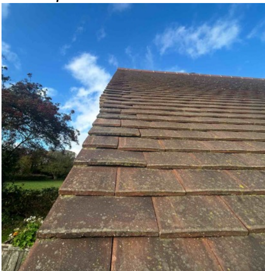
Plate 6: Gaps Under Tiles
