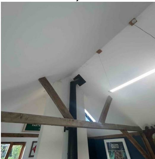
Plate 5: No Suitable Roof Void
