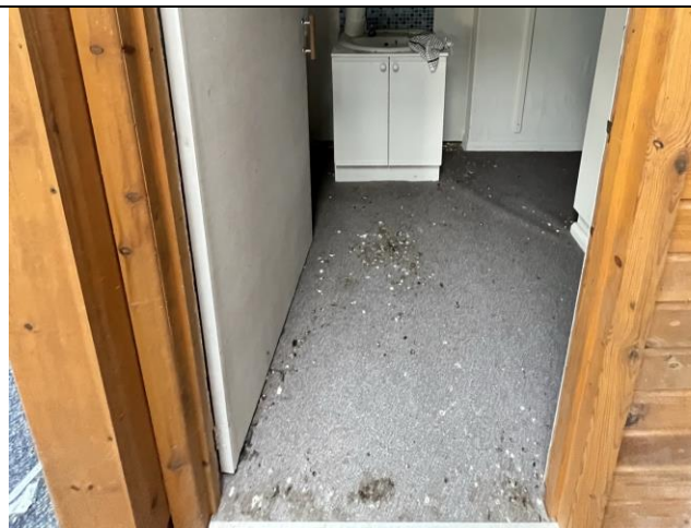
Photograph 4: bird droppings within the farm building.
