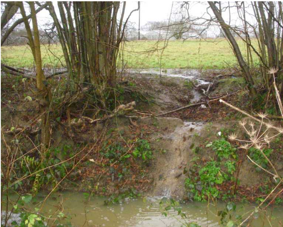
Fig 6 Standing water at Sandgate south side and heavy flowing, excess run off into south side ditch.
