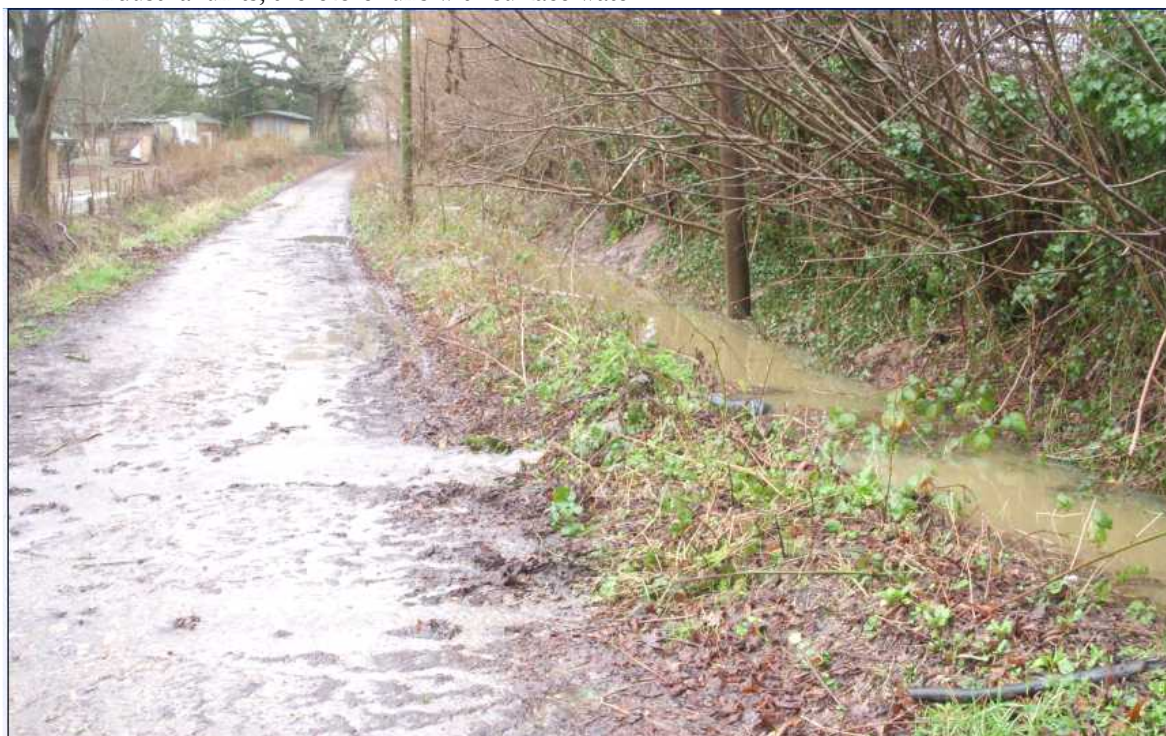
Fig 7 Sandgate - ditch to north of Hollands Lane unable to cope. Surface flooding to Hollands lane
