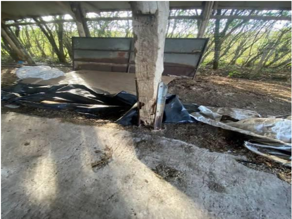
Evidence of several of the structural uprights dangling from the rafters.
