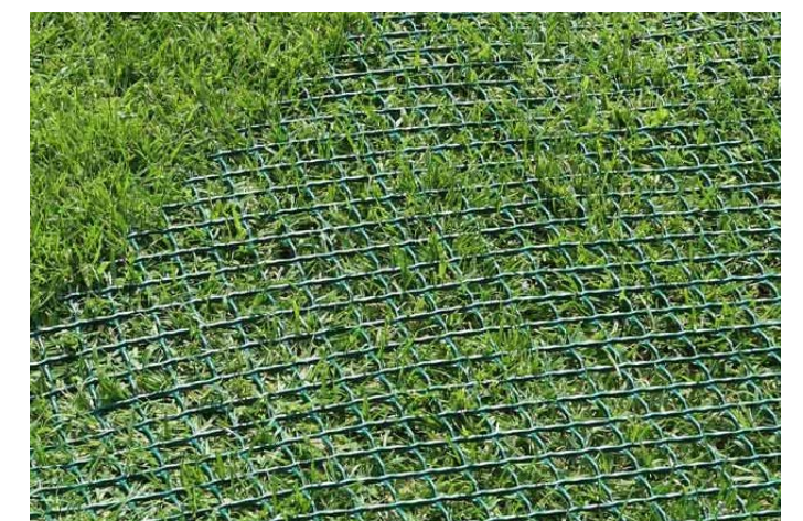
Grass reinforcement mesh parking area
