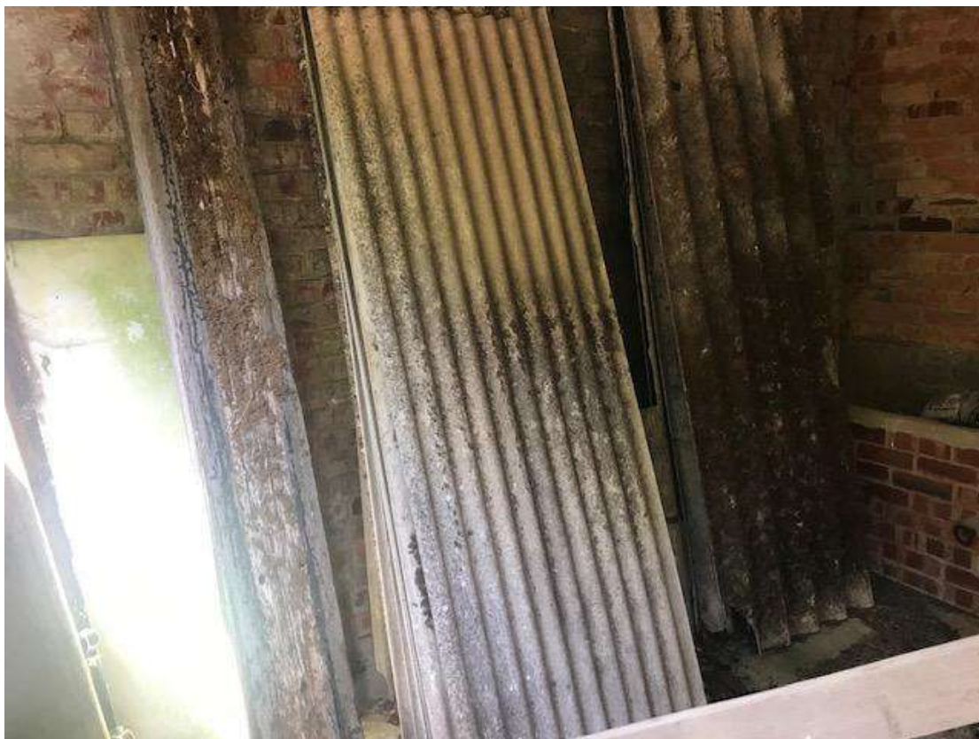
Roof cladding, possible asbestos contaminant
