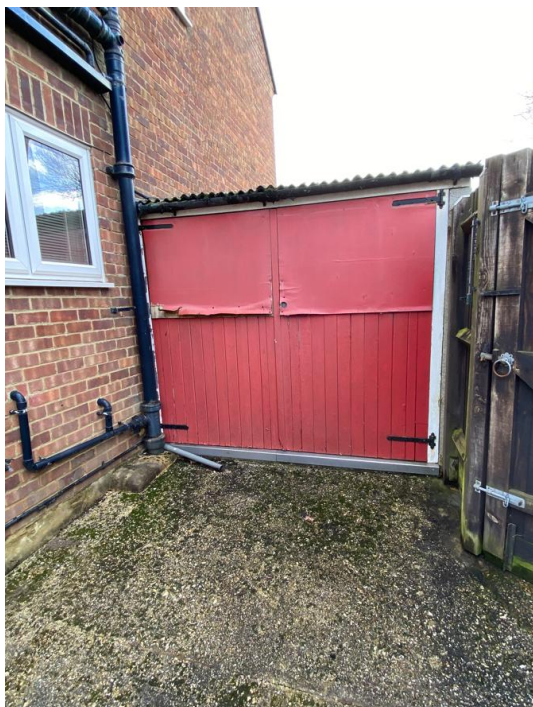
Rear view of dilapidated garage
