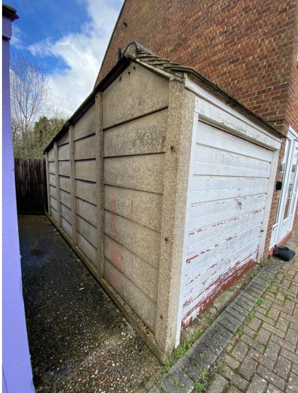
Pre-fab dilapidated garage
