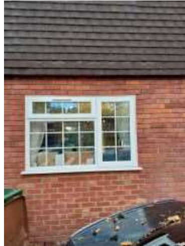
No Lintel above bottom right window
