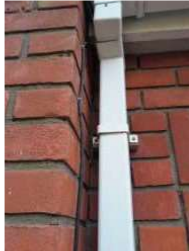
No separation on left side of porch
