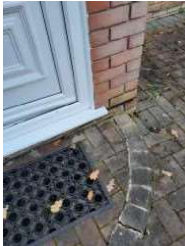
Separation between cill and brickwork
