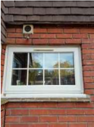
No Lintel above window next to porch
