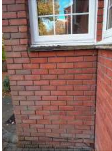
Porch joining main building. The brickwork has slipped off DPC and no separation between the porch and main house on the right side.
