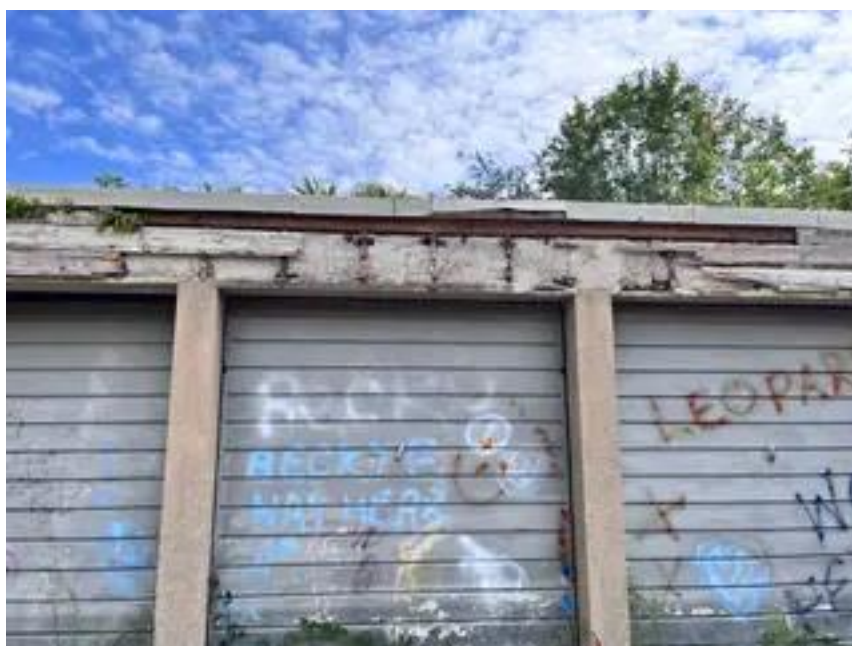
Photograph 5. The low potential feature on Building 2.
