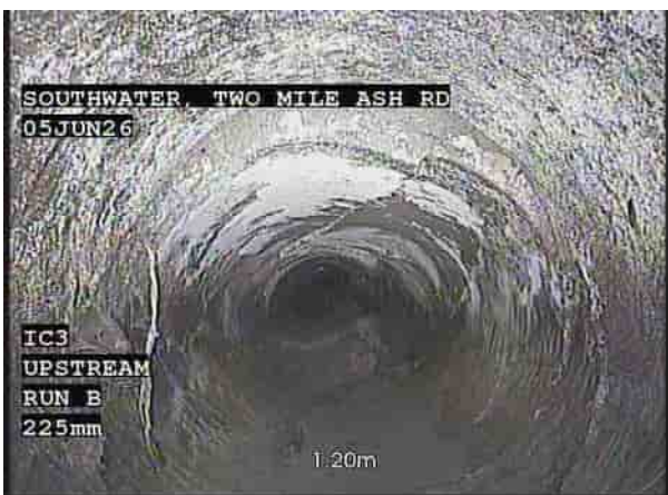
3, 00:00:25, 1.20 m Settled deposits, fine, 10% cross-sectional area loss, start
