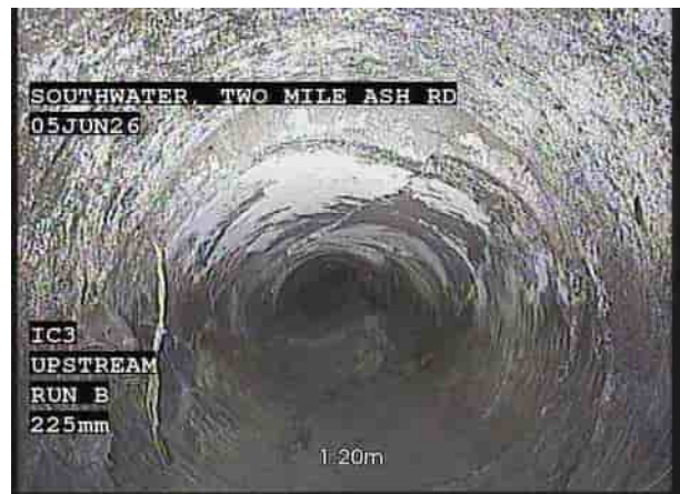
2, 00:00:18, 1.20 m Deformed sewer or drain, 20%, start
