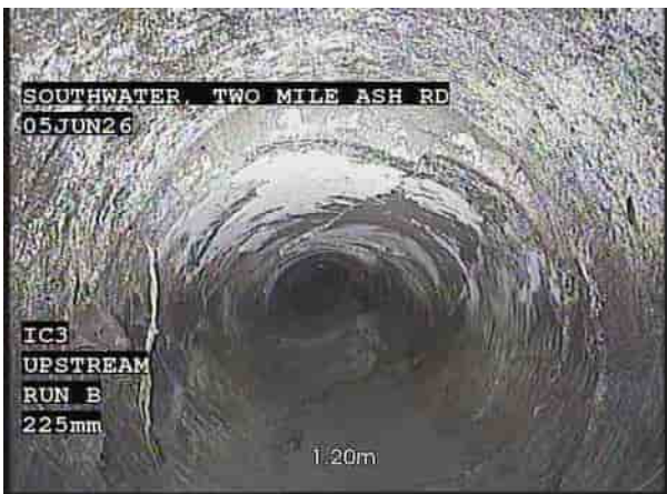
1, 00:00:12, 1.20 m Fractures, multiple from 12 o'clock to 12 o'clock, start
