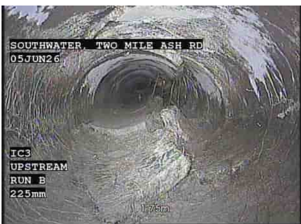
5, 00:00:49, 1.75 m Broken pipe from 12 o'clock to 12 o'clock
