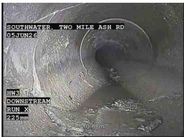
3, 00:01:02, 0.88 m Fractures, multiple from 12 o'clock to 12 o'clock
