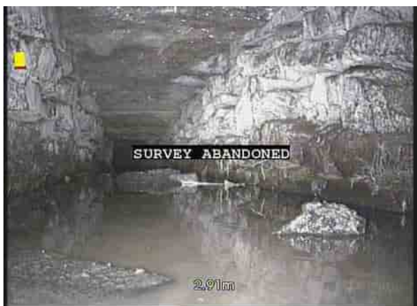
1, 00:00:29, 2.91 m Survey abandoned, Unable to pass
