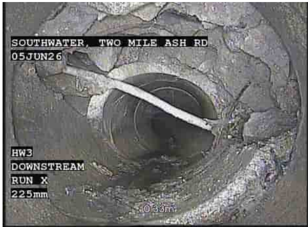
1, 00:00:32, 0.33 m Void visible beyond defect
