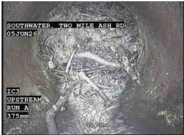
1, 00:04:00, 46.15 m Settled deposits, coarse, 100% cross-sectional area loss
