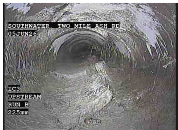
4, 00:00:42, 1.75 m Deformed sewer or drain, 50%
