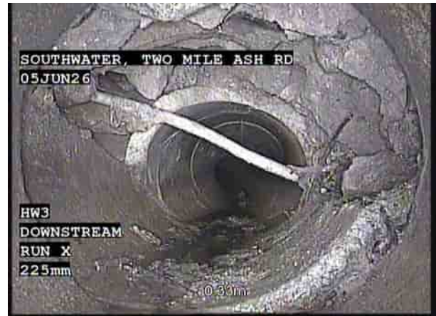
2, 00:00:40, 0.33 m Broken pipe from 10 o'clock to 4 o'clock
