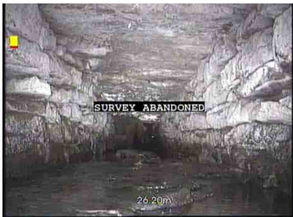
3, 00:04:55, 26.20 m Survey abandoned, Unable to continue
