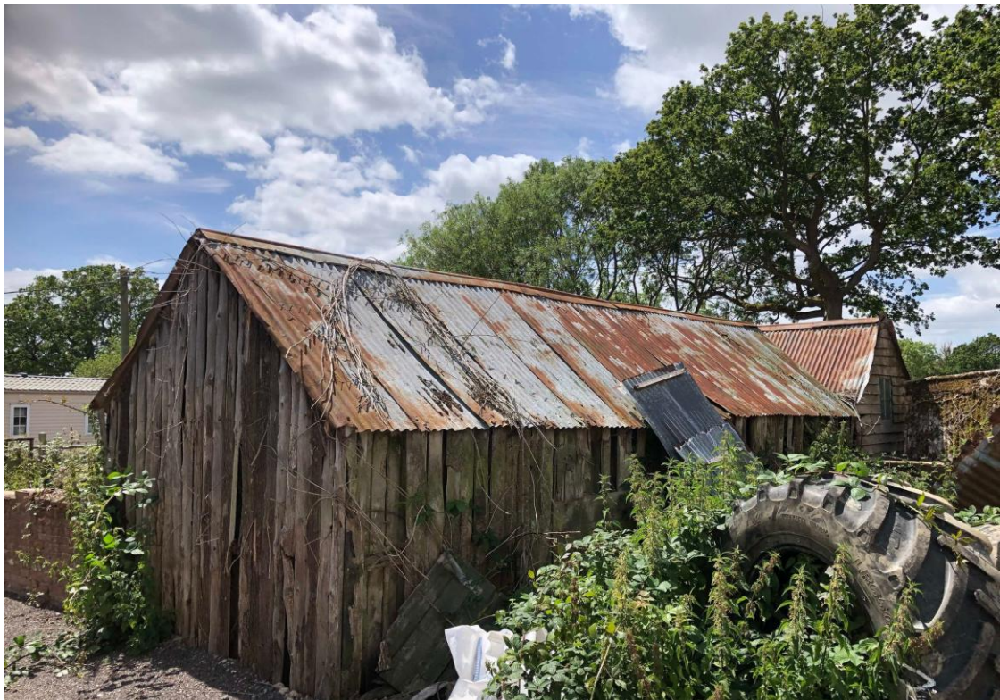
Fig 6: The improvised building is poorly constructed using tree trunk/branch cladding and a corrugated roof. On balance, the building is thought to be capable of replacement, subject to appropriate design.
