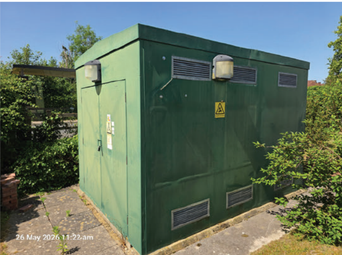
The electricity substation from the car park.
