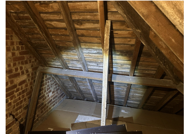
Figure 1a: Internal void of B1
