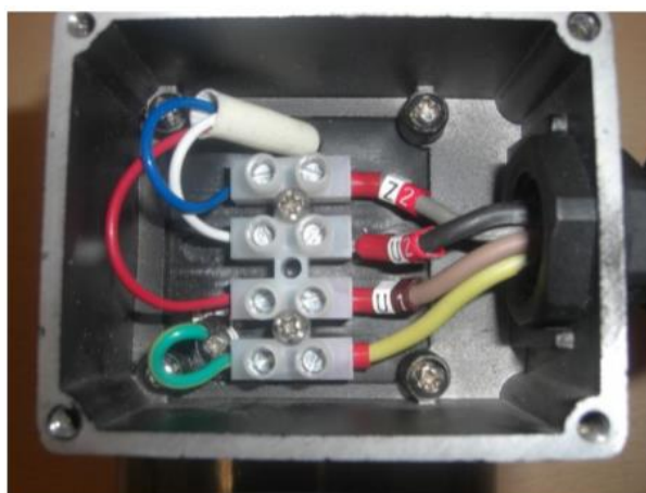
Motor Terminal Box
