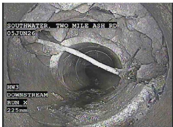
1, 00:00:32, 0.33 m Void visible beyond defect
