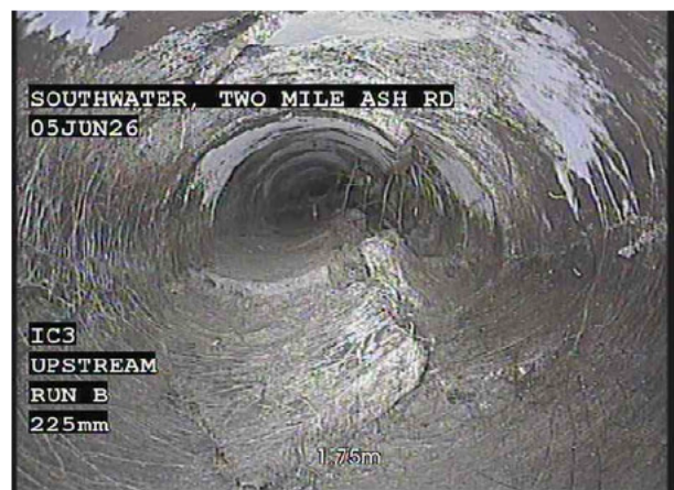
4, 00:00:42, 1.75 m Deformed sewer or drain, 50%
