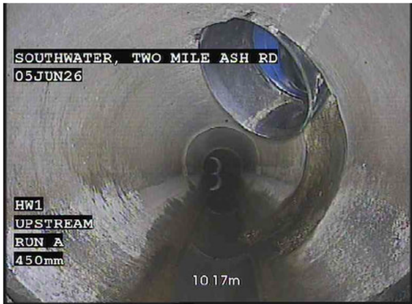
1, 00:00:57, 10.17 m Connection defective, connecting pipe is intruding at 2 o'clock, 150mm dia, intrusion: 20%
