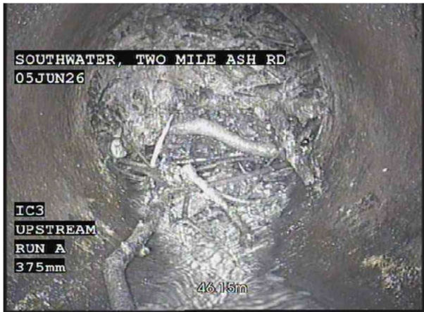
1, 00:04:00, 46.15 m Settled deposits, coarse, 100% cross-sectional area loss
