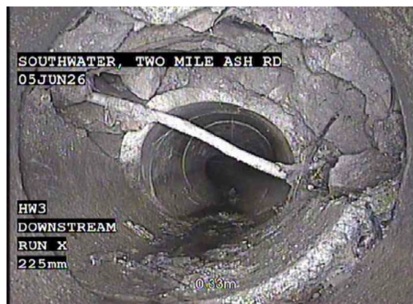
2, 00:00:40, 0.33 m Broken pipe from 10 o'clock to 4 o'clock
