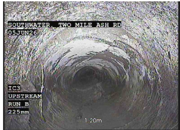
2, 00:00:18, 1.20 m Deformed sewer or drain, 20%, start
