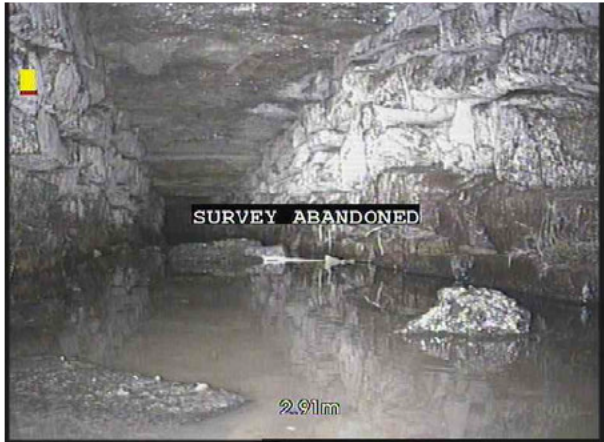
1, 00:00:29, 2.91 m Survey abandoned, Unable to pass
