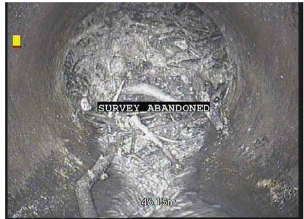
2, 00:04:08, 46.15 m Survey abandoned, At OF2 chamber - debris filled
