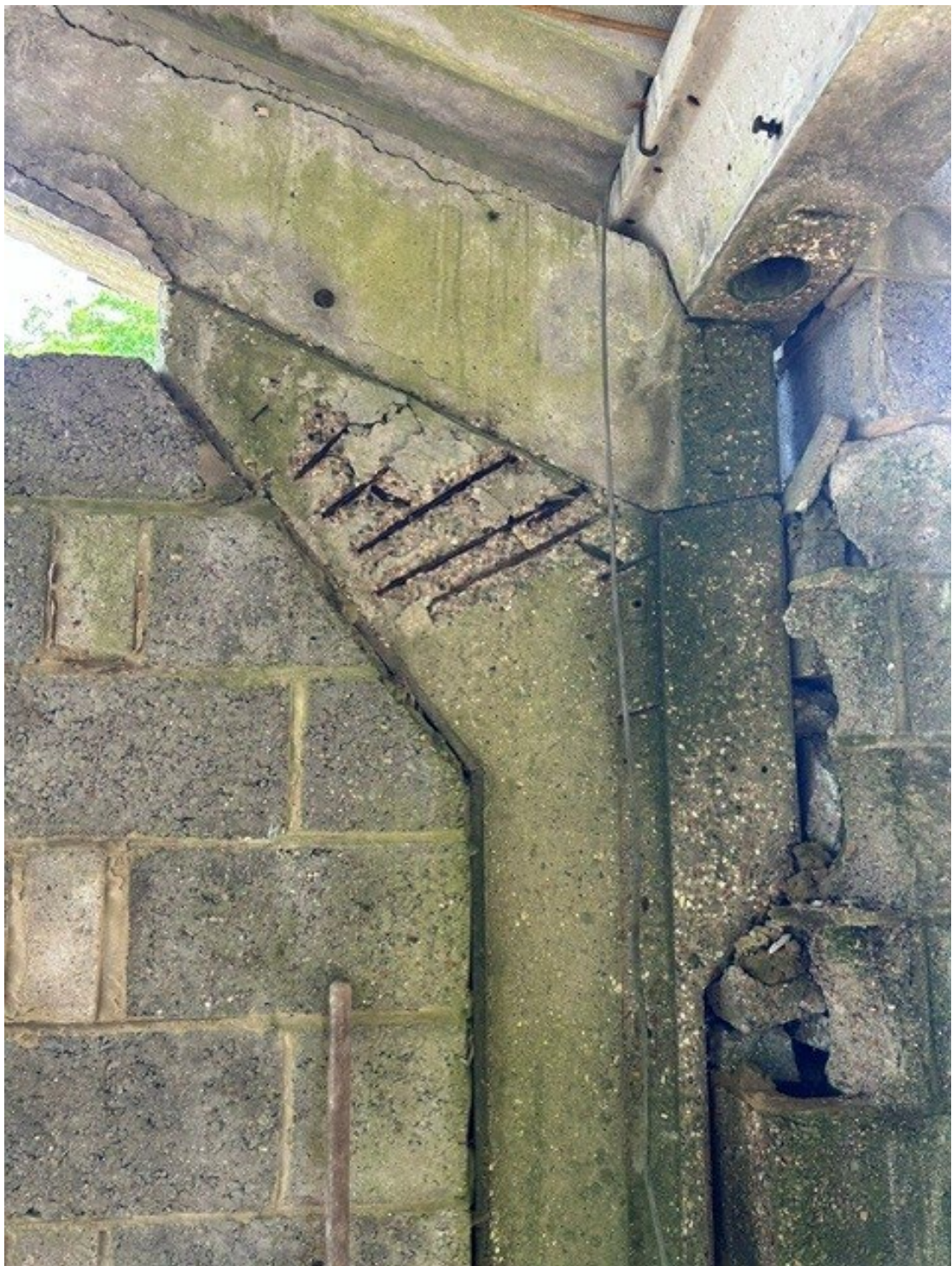
2 Spalling on face of column
