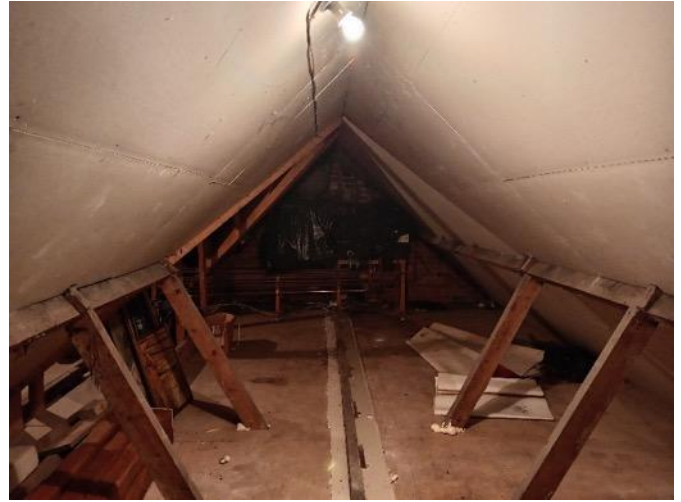
Photograph 2. Internal loft space of B1, location of bat droppings
