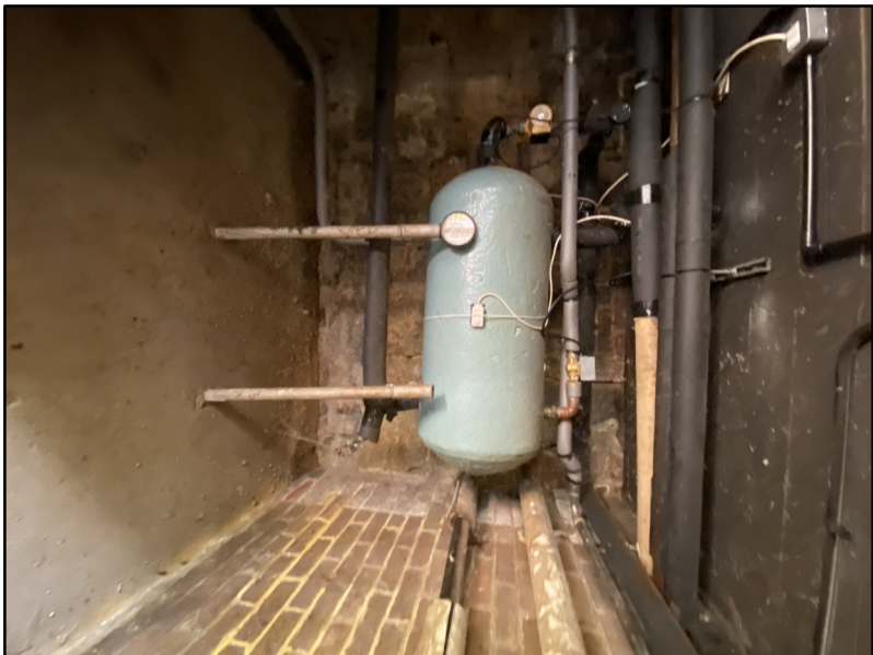
Boiler room RB.04
