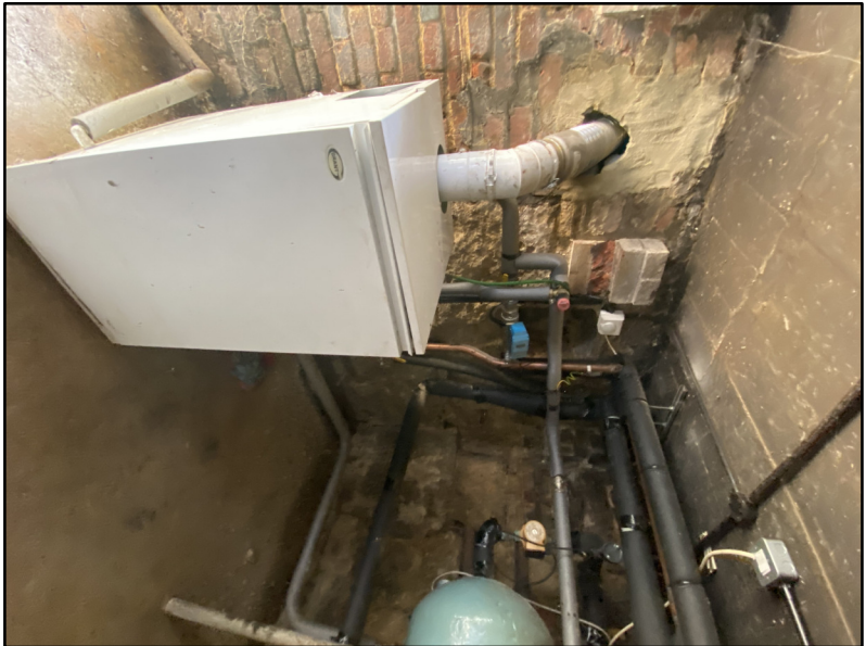
Boiler room RB.04
