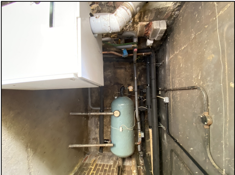
Boiler room RB.04
