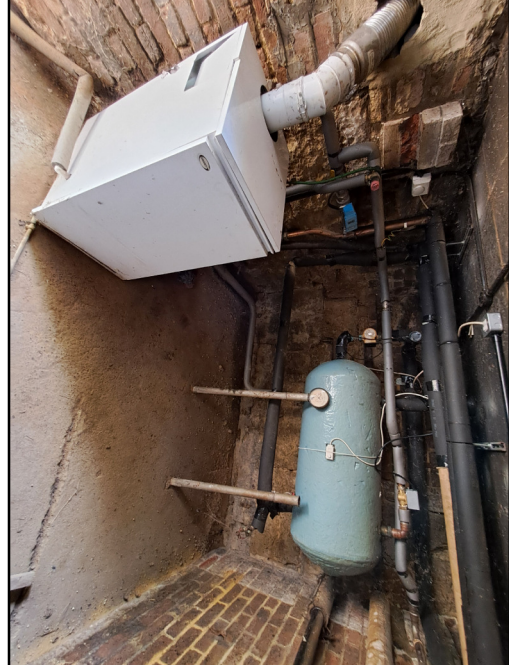
Boiler room RB.04
