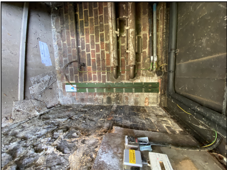
Boiler room RB.04
