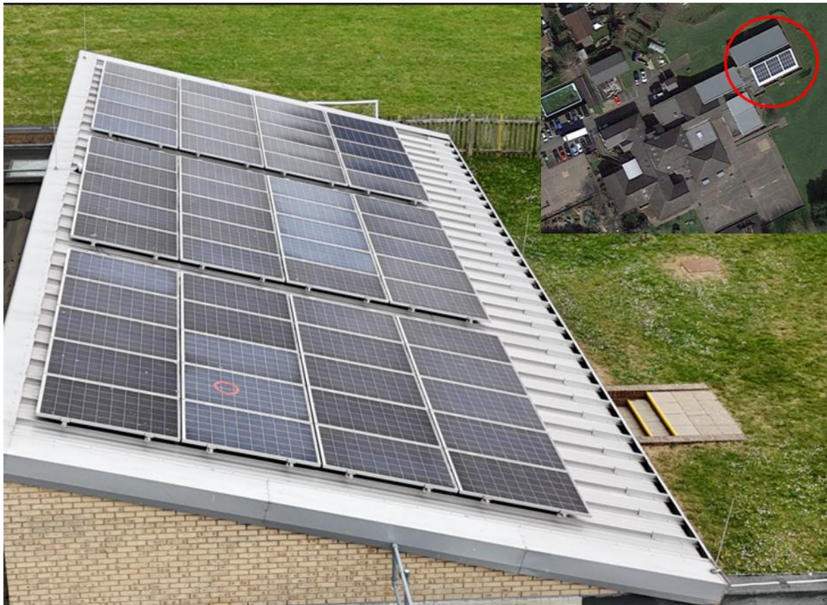
St Marys C of E Primary School: Existing solar PV array. Inset aerial photo shows location of roof.
