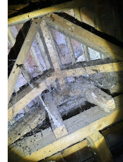
Cobweb accumulation around apex ridge beam of B1.
