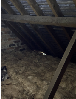
Light ingress from gaps in roof tiles.
