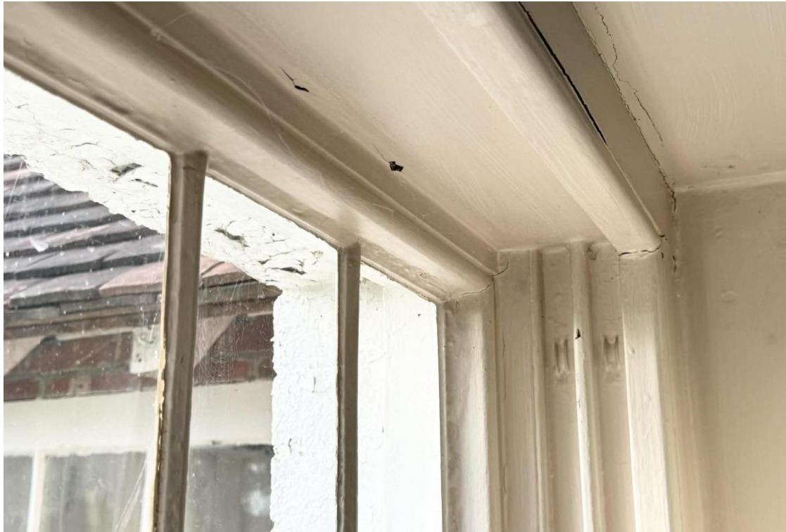
Fig 1: Behind the metal windows sit vacant runners with pulleys, indicating sash windows once sat there.
