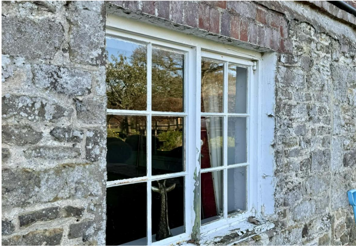
Fig 8: The windows are in a poor state of repair and are capable of replacement, subject to appropriate design.
