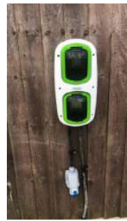
Electric vehicle charging point
