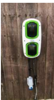
Electric vehicle charging point
