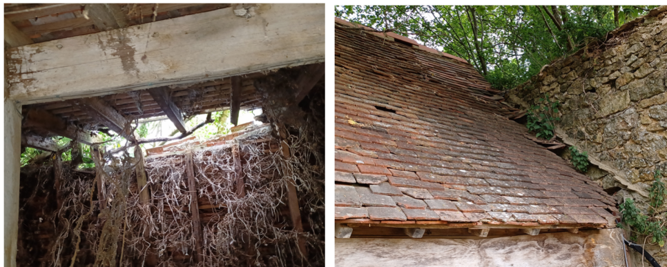
Figure 1: Images showing condition of the roof covering
