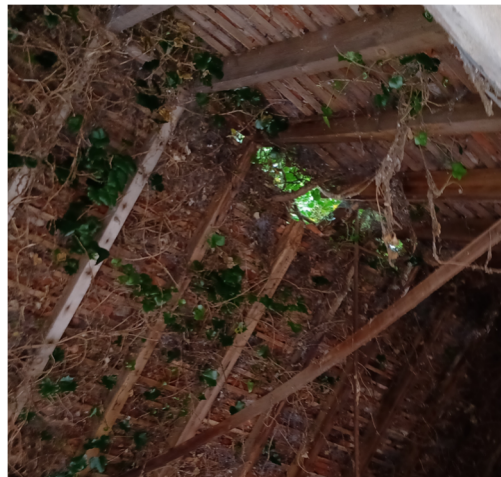
Figure 2: Image showing the ends of the commons rotten through
