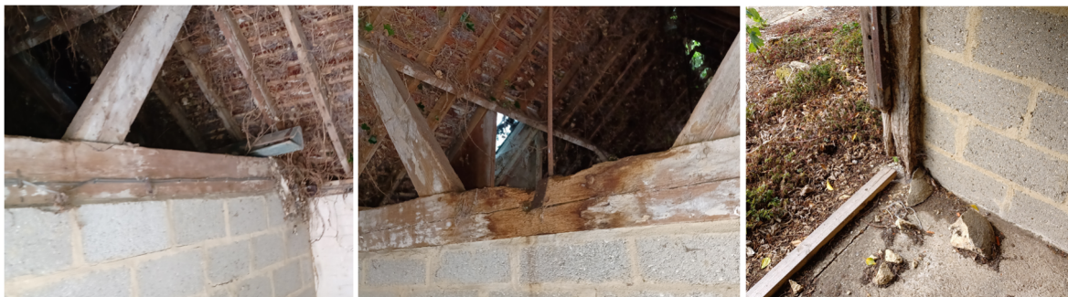
Figure 3: Images showing the condition of the main frames
