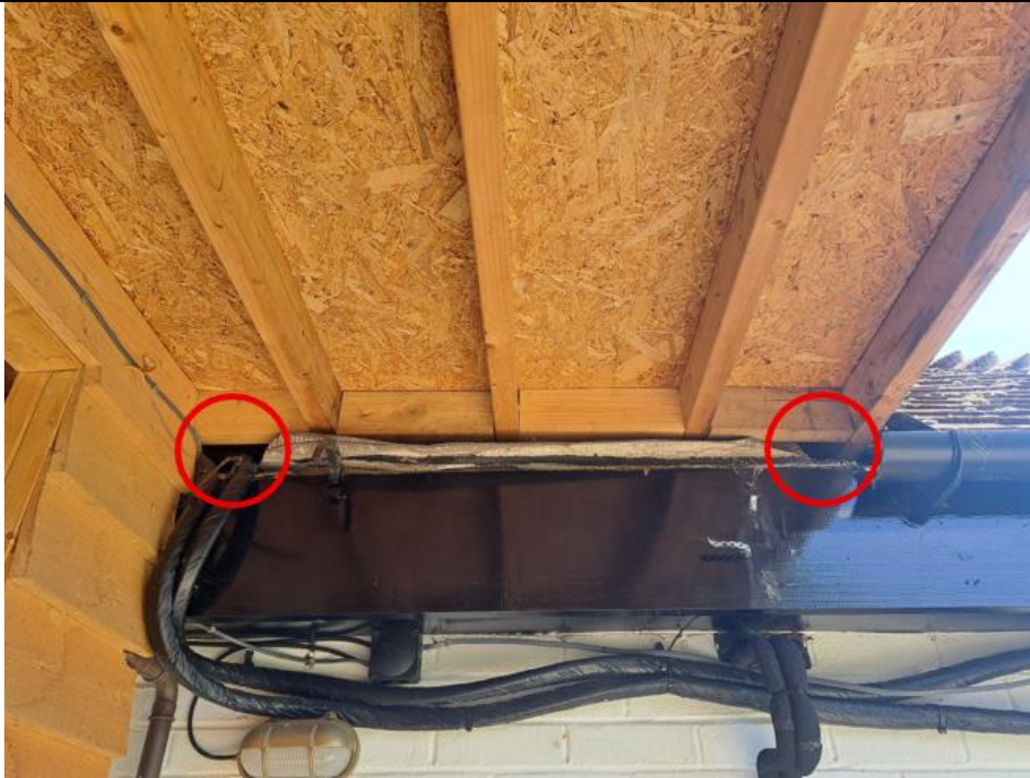
Potential roosting features at join between timber canopy and main building roof.
