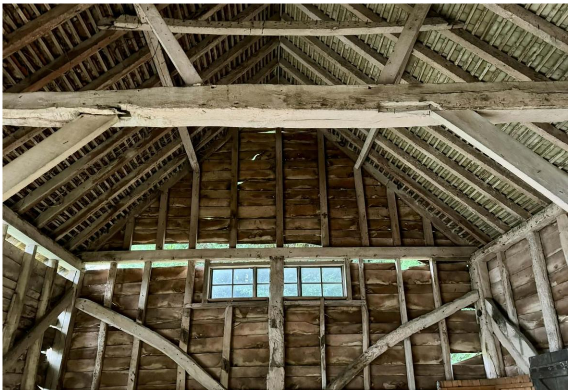
Fig 8: Although the former tithe barn has been re-roofed and has modern rafters, the main timber frame itself remains, for the most part, historic fabric with many original oak posts, including traditional scarfing joints.
