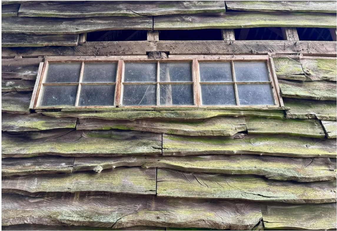
Fig 7: A timber casement window on the side elevation is placed externally behind the central timber post and is reflective of the evolution of the former tithe barn. This will be retained as part of the proposed design.
