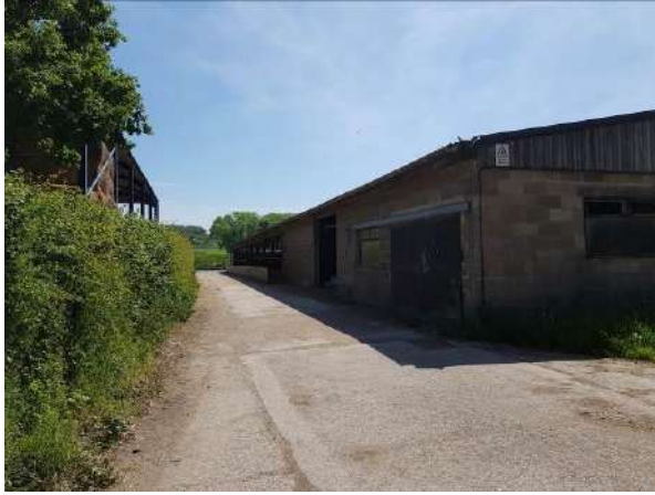
Photo 1: Northern and western elevations of B2, with southern elevation of B1 in left-side of photo.
